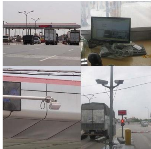
Fig. 4 ETC lane in Long Thanh – Dau Giay Expressway
