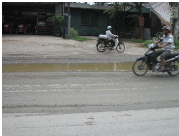
Fig. 7 Rutting, water and dust on road
